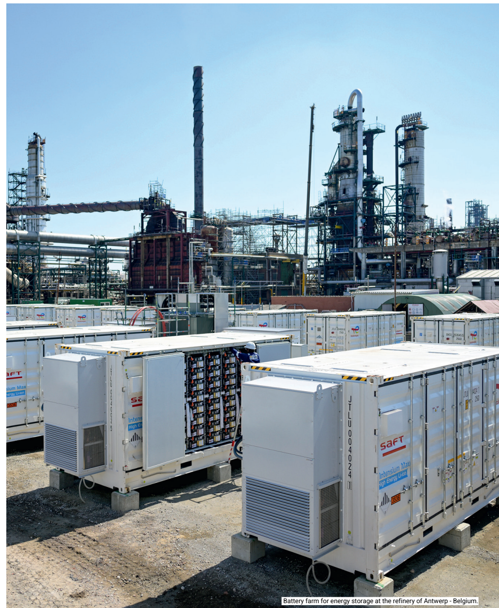
Battery farm for energy storage at the refinery of Antwerp - Belgium
